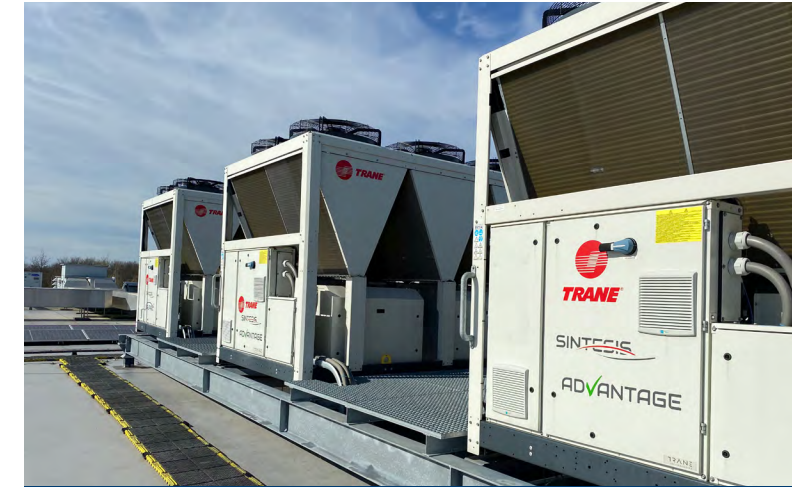
In 2022, our Kerkrade team began the conversion to a zero-natural gas facility, installing heat pumps that are far more energy-efficient than fossil fuel-fired boilers. In 2023, we completed the transition across the campus.
